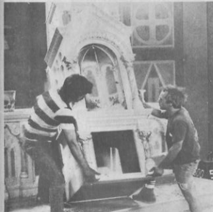
Larry Weaver (left) and Lance Alletzhauser remove a section of the church alter to be shipped through their architectural antique business to southern buyers. The church had been vacated for several years (below) as the parish is planning a new building at an adjacent site. In the bell tower (below, right) names of repairmen and bell-ringers remained as one last touch of sentimentality before the actual demolition began this week. (Arick Sonneborn photos)
